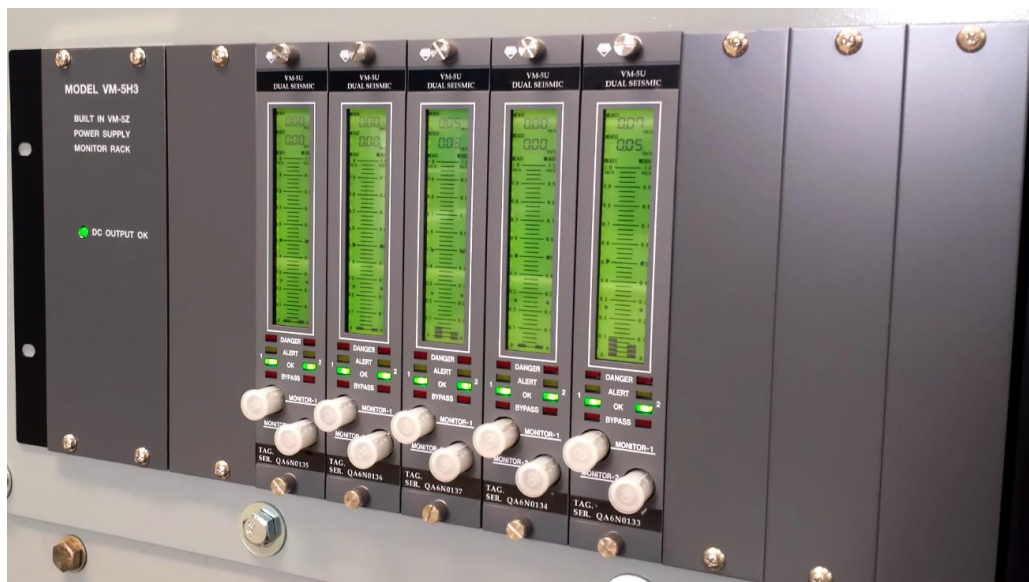
Picture 1 – One of the VM-5 Monitors installed at DuPage Water's Elmhurst Station
